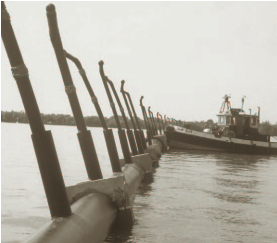
Figure 16: Typical vertical riser construction. The all polyethylene riser is socket fused to the line of SCLAIRPIPE and an additional section of larger diameter SCLAIRPIPE is placed over the riser and extruder welded to the outfall pipe for reinforcement.
