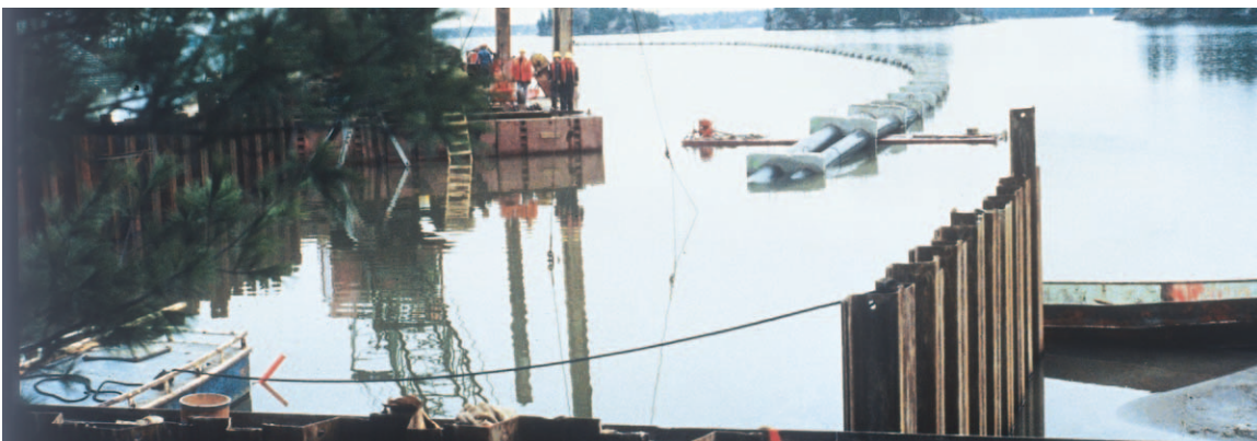
Figure 13: Sinking of a SCLAIRPIPE outfall line at Gravenhurst, Ontario. Pipe was lifted at a point off shore to induce a water pocket in the line. This controlled the rate of sink by preventing water from running the full length of the pipeline.
