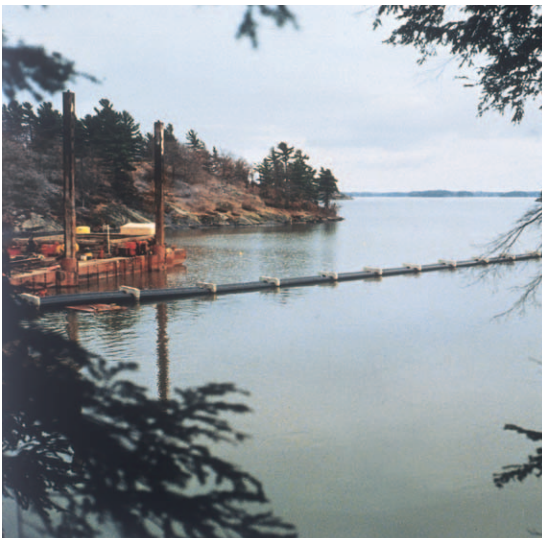
Figure 6: Floating SCLAIRPIPE line complete with concrete weights being prepared for the sinking procedure.
