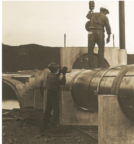
Figure 5: Use of a skidway to convey 40" pipeline of SCLAIRPIPE to the water, allowing the weights to be moved along with the pipe with minimum drag.
