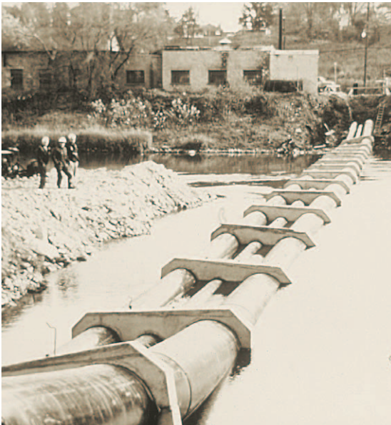
Figure 4: Triple inverted sewage siphon of 20, 28 and 40 inch SCLAIRPIPE being installed in Galt, Ontario. Concrete weighting collars, embracing the three pipes, were attached on shore and the lines were floated into position and gradually sunk in a single operation.
