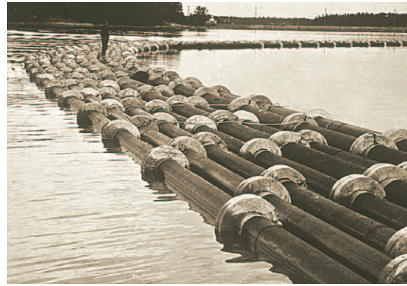
Continuous fused lengths of SCLAIRPIPE weighted with cylindrical concrete collars and stored floating in the water.
