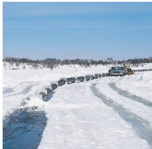
Figure 21: Installation of 28" water intake line of SCLAIRPIPE at Lac-des-Ecorces, Quebec. The pipe was weighted with concrete collars and allowed to sink through a cut in the ice.
