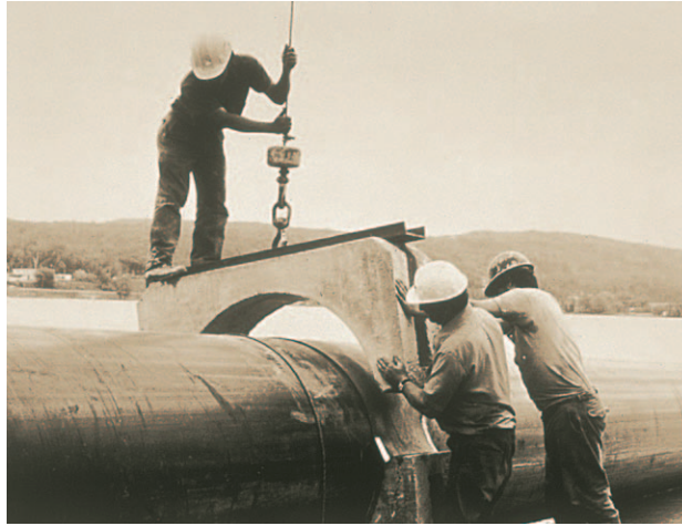
Figure 1. Ballast weights being attached to a 48" SCLAIRPIPE line on shore, prior to launching of the pipe.
