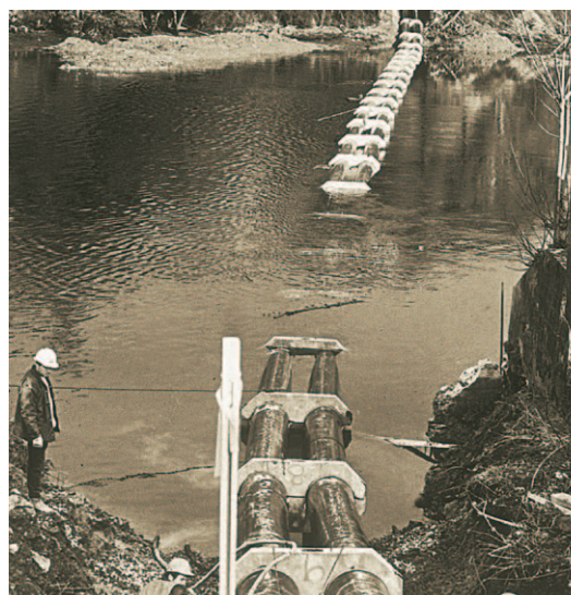
Figure 3: Installation of 24" SCLAIRPIPE for twin sewage siphon in Victoria, B.C. Specially designed concrete weighting collars, embracing the two pipes, were attached on the water and the lines were floated into position and gradually sunk.
