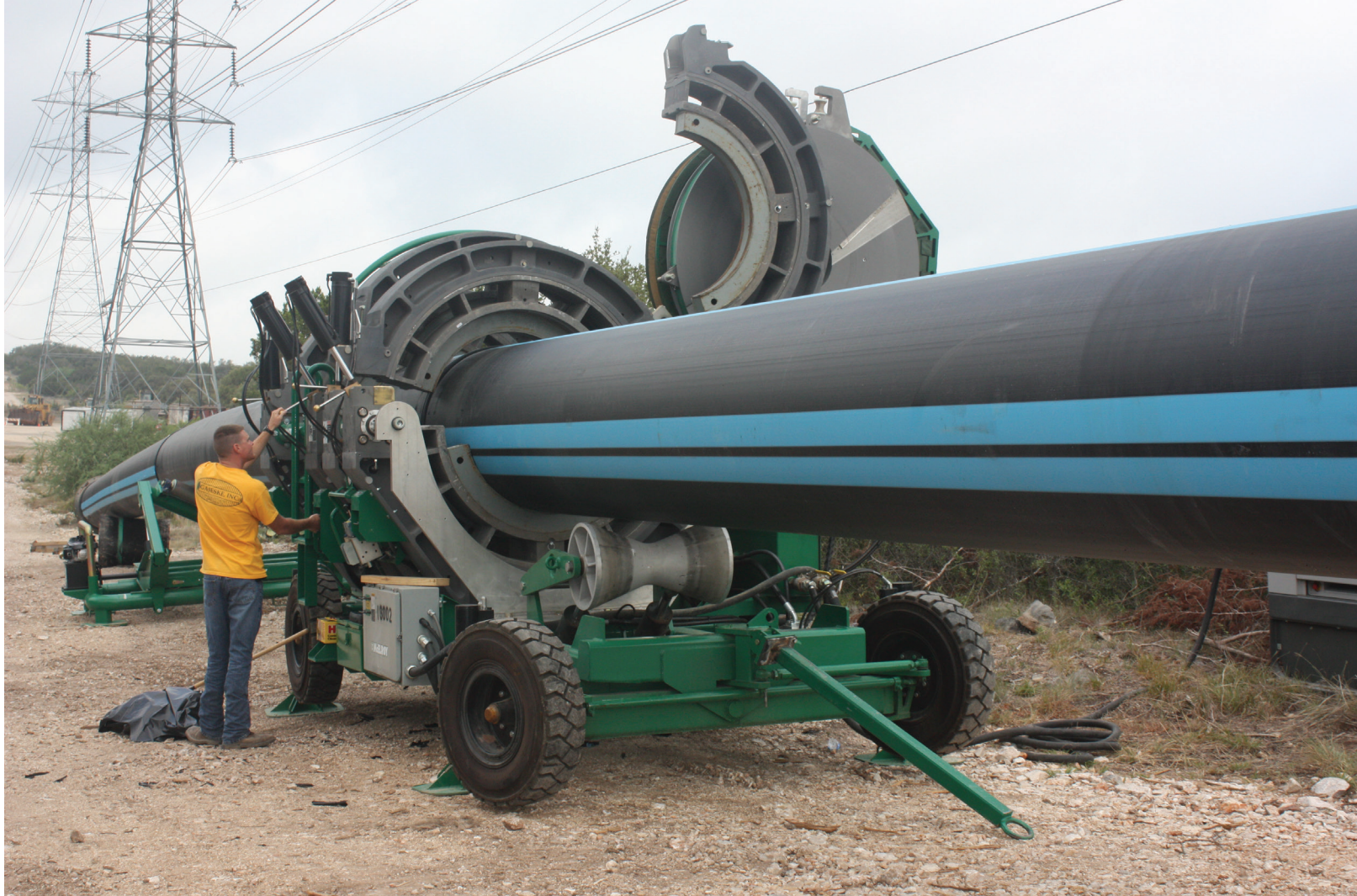
Above: Heat fusing sections of PE4710 HDPE pipe provide a leak-free system. Opposite page: Long runs of PE4710 HDPE pipe can be installed in a trench or by a number of trenchless methods.
